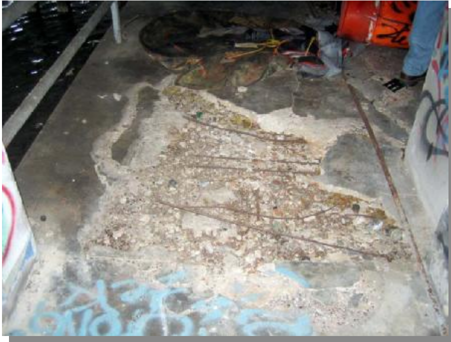
60- Lower Level Walkway Slab Deterioration
