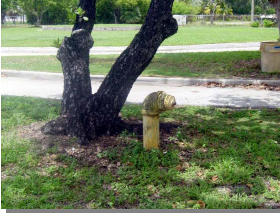
1- Fire Department Connection
