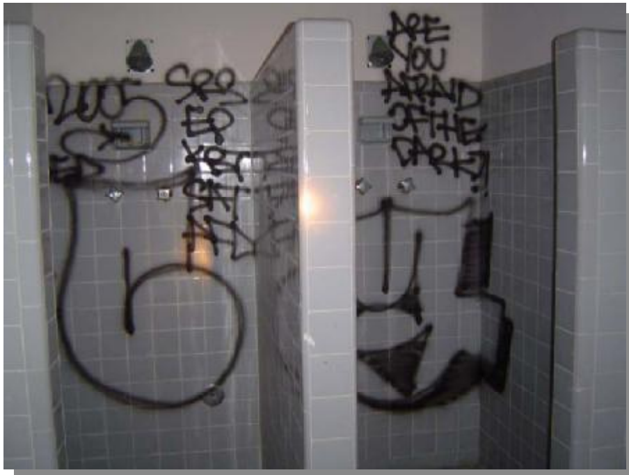
24- Tile with Possible Lead Content May Need to be Abated
