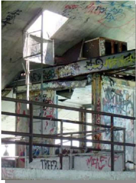
70- Over Head Control Booth with Steel Structural Beam Penetrating Concrete Structure
