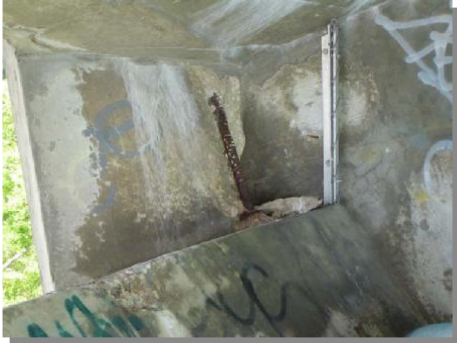
68- Main Column Deterioration
