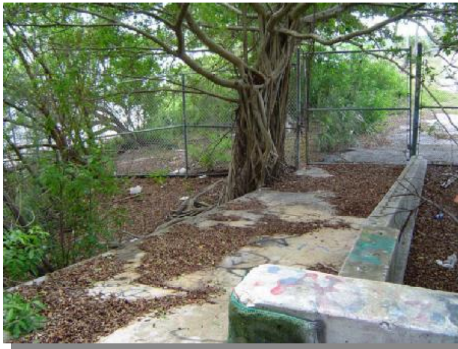
14- Ramp Access at Ground Level – No Guardrails and Handrails
