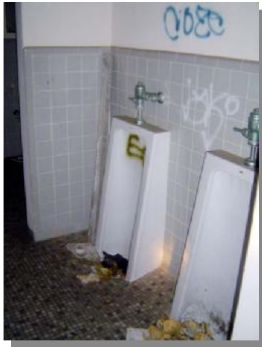
39- Plumbing Fixtures with Debris
