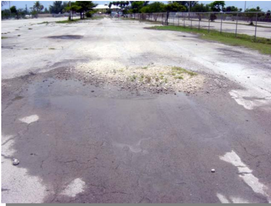
2- Parking Area Paving Deterioration
