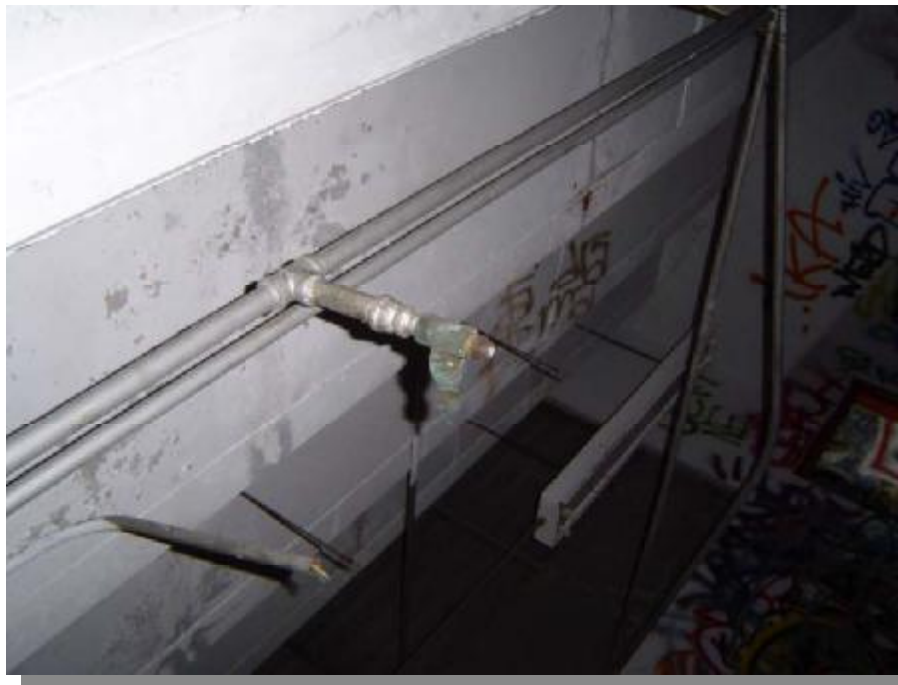
44- Potable Water Cold Supply
