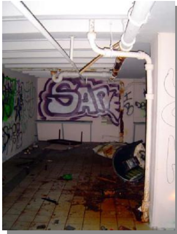
37- Cast Iron Sanitary Line Deterioration
