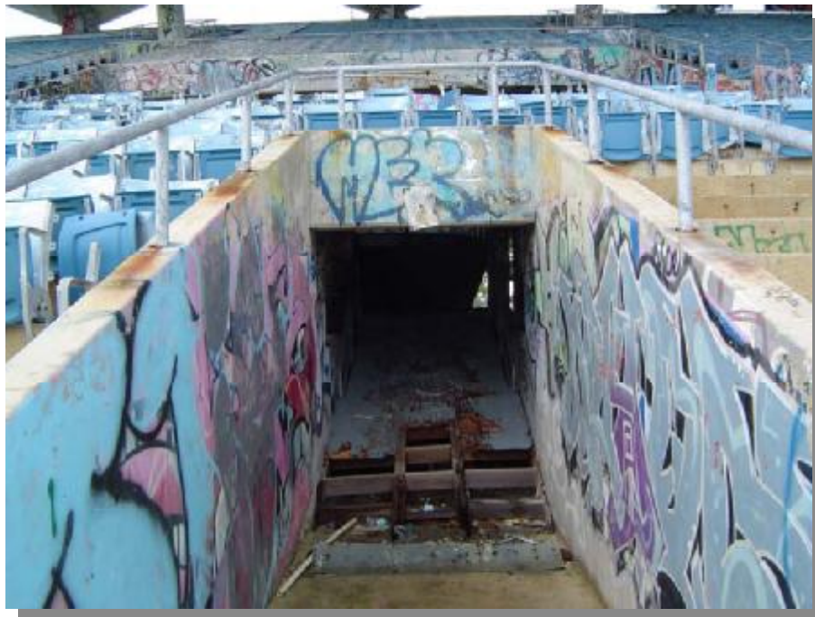
22- Ramp to Lower Level – No Guardrails and Handrails
