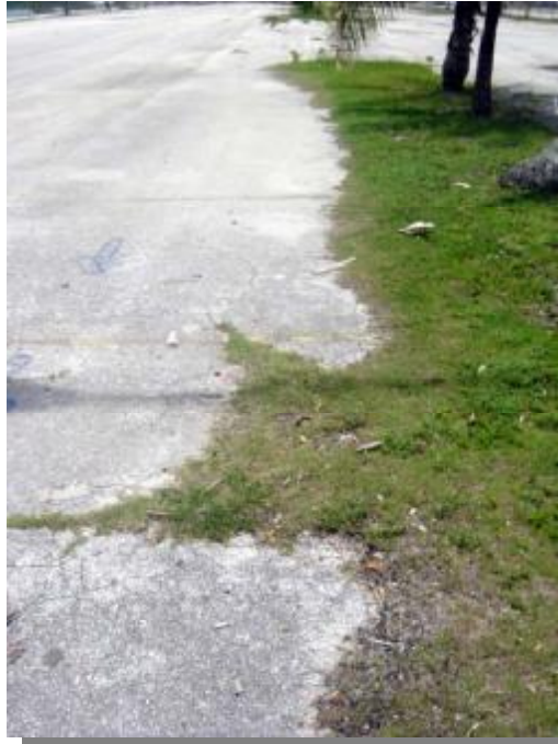
3- Landscape Area Encroaching Into Parking Area
