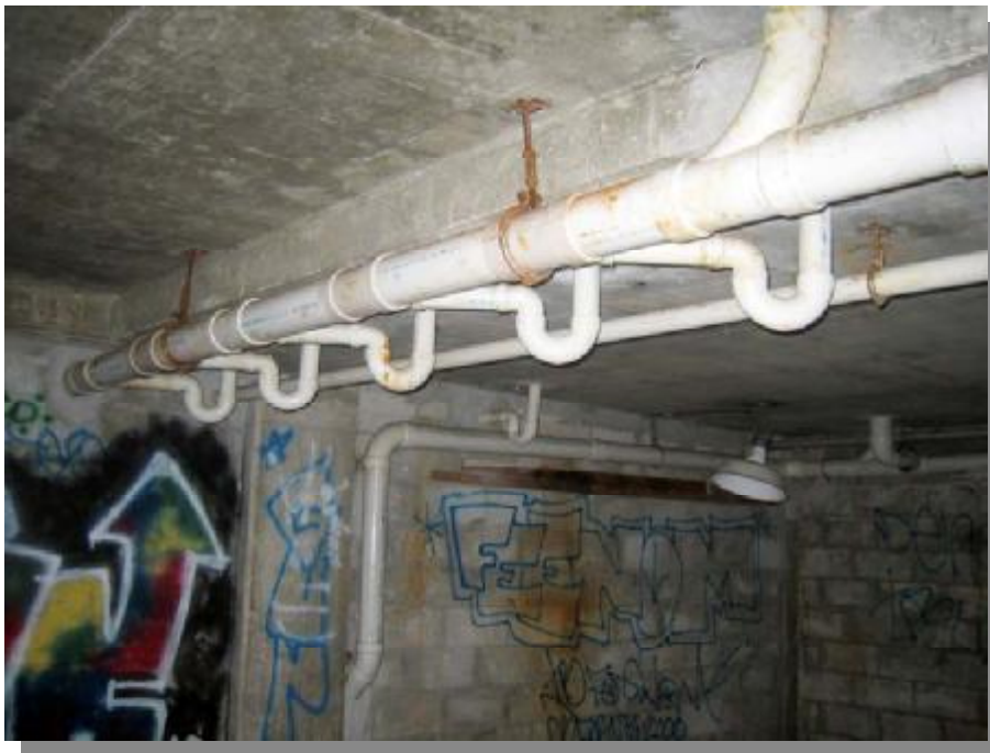
34- Sanitary Piping PVC Retro Fit and Missing Pipe Supports
