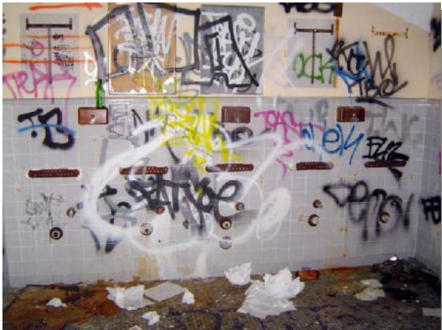
46- Restroom with All Fixtures Stolen
