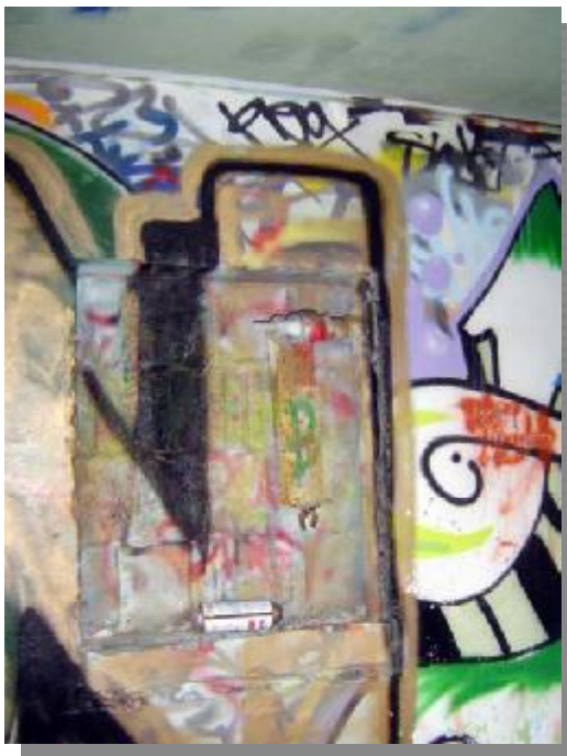
42- Disassembled Fire Hose Cabinet
