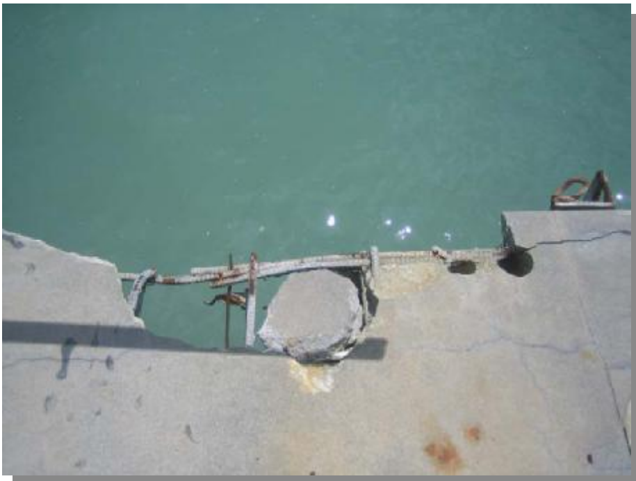
61- Lower Level Slab Deterioration
