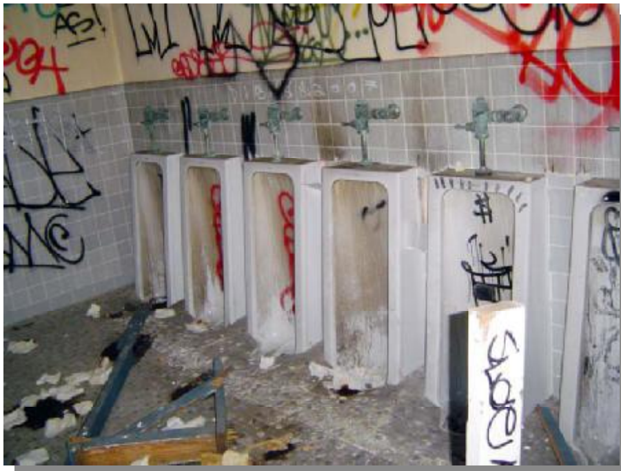
48- Plumbing Fixtures with Debris
