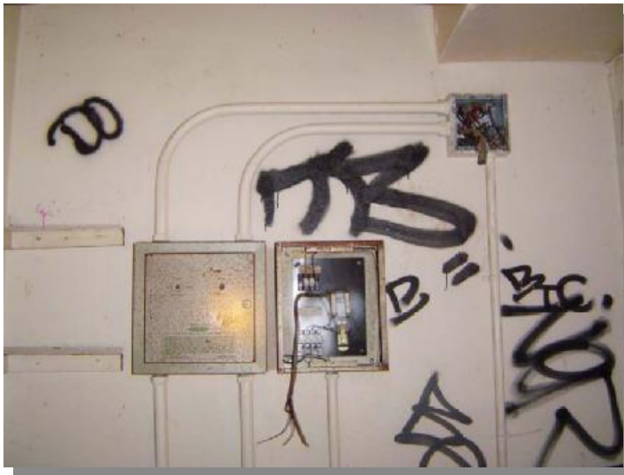
54- Open Junction Box and Disassembled Disconnect
