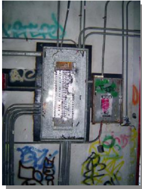
55- Disassembled Electrical Panel
