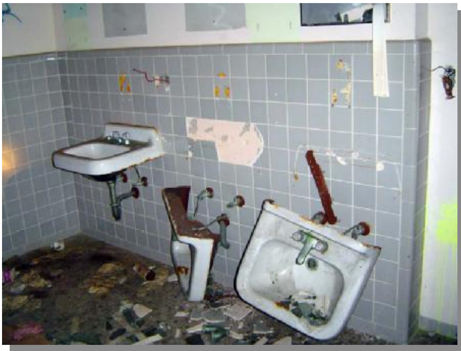
38- Plumbing Fixture Damage
