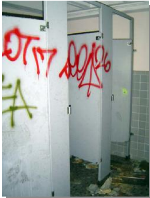
23- Rest Room Stalls, No Handicap Accessibility
