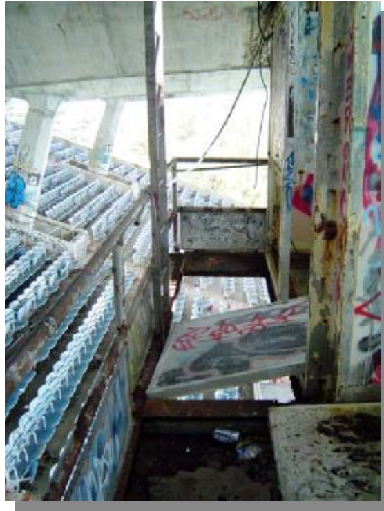
72- Control Booth Structure Deterioration
