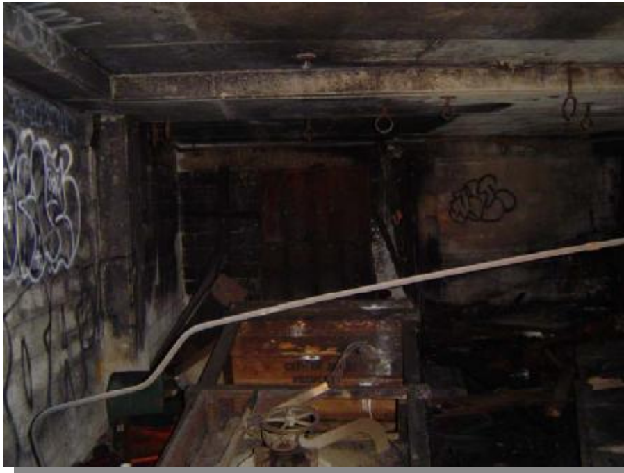
19- Area with Fire Damage
