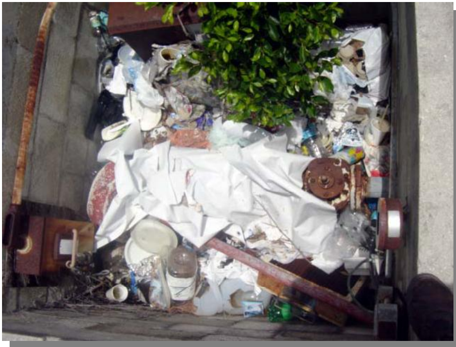
8- Water Service Enclosure
