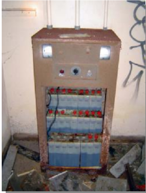
25- Hazardous Material Battery Back Up System
