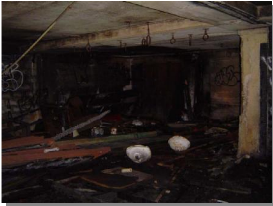
18- Area with Fire Damage
