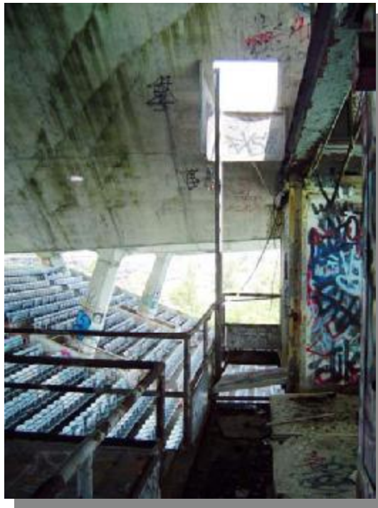
71- Control Booth Structure Deterioration
