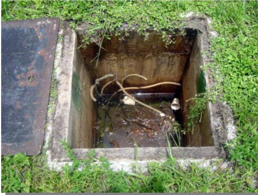
7- Equipment Box Equipment Stolen
