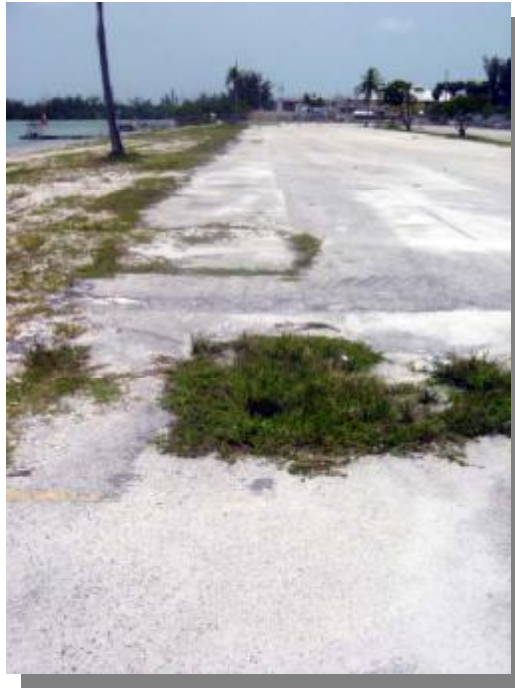
5- Parking Area Deterioration
