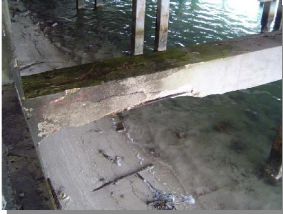
62- Concrete Beam Damage
