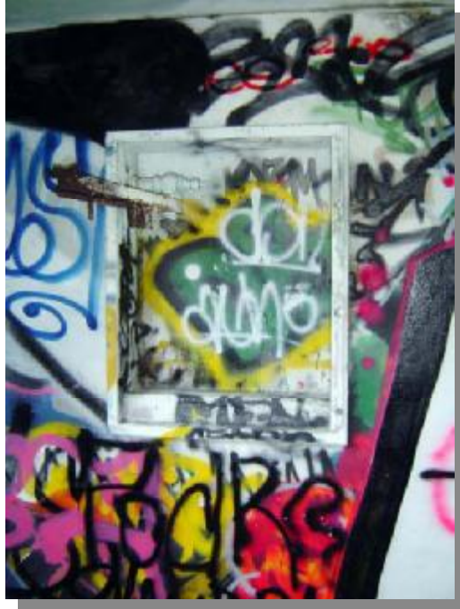
41- Disassembled Fire Hose Cabinet
