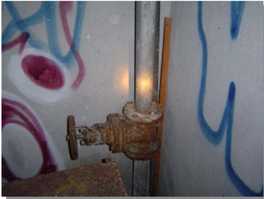
36- Fire Hose Riser
