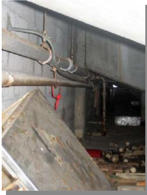
35- Air Handling Units in Crawl Space
