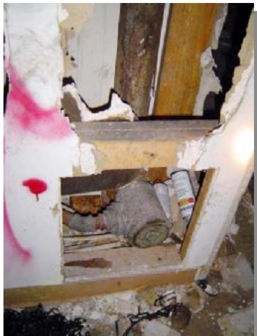
40- Cast Iron Sanitary Piping Deterioration
