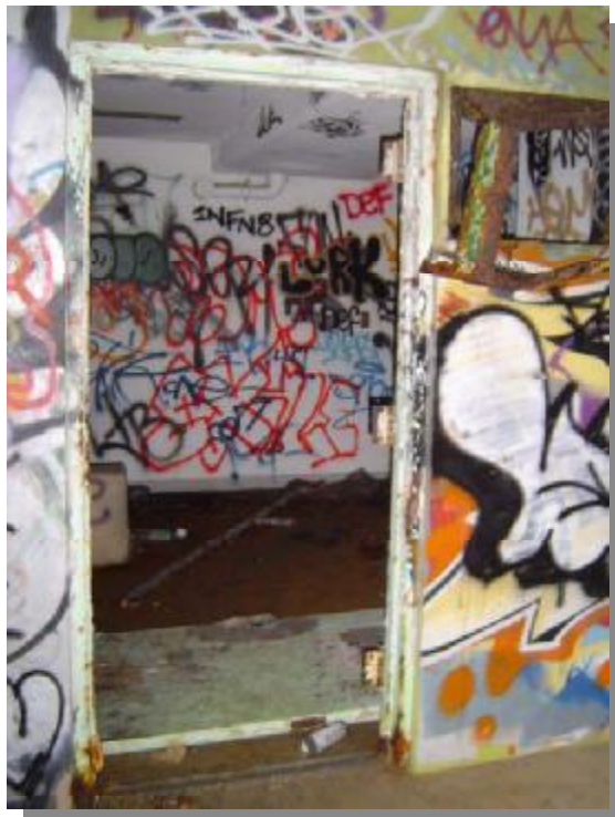
16- Typical Building Condition
