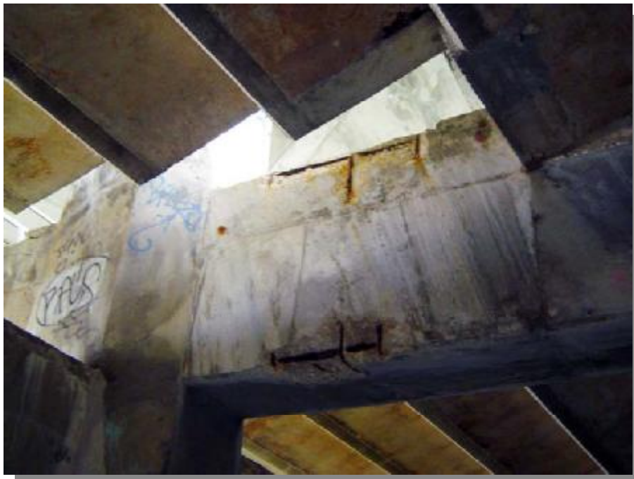
65- Main Support Beam Deterioration
