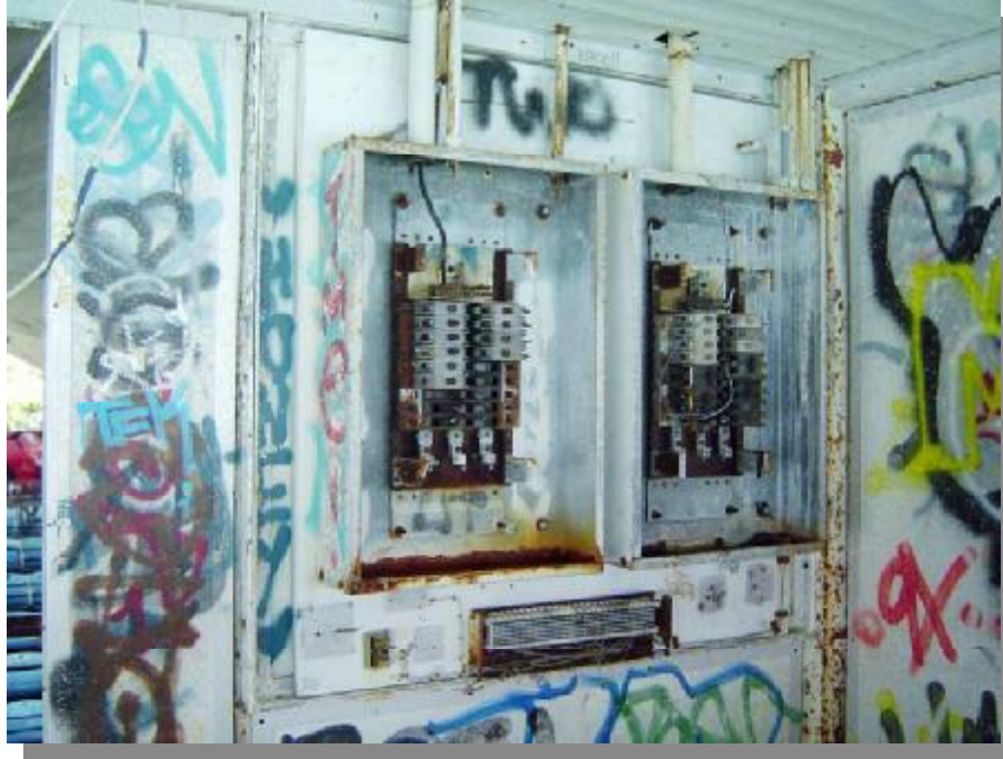
57- Disassembled and Deteriorated Electrical Panels
