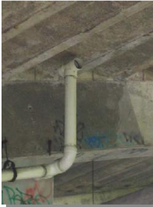
33- Sanitary System Vented Below Grand Stand Seating
