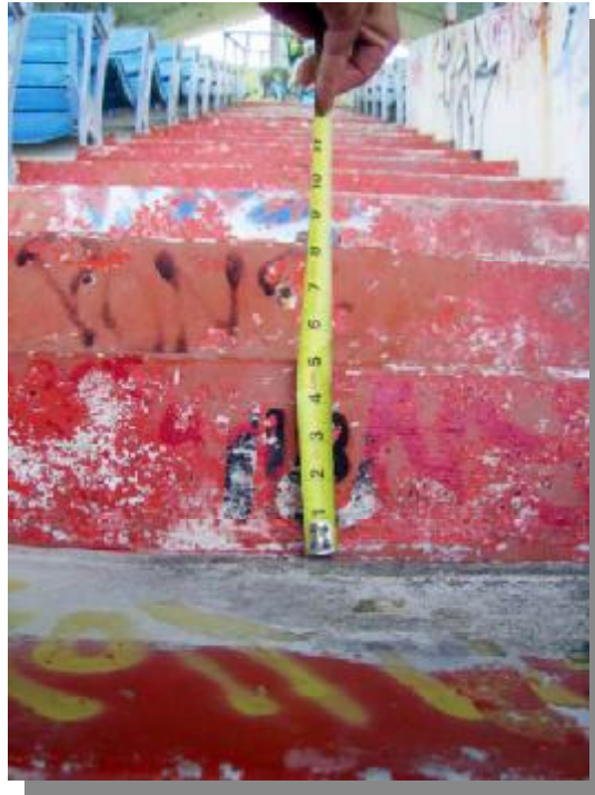
11- Stair Riser 5" High
