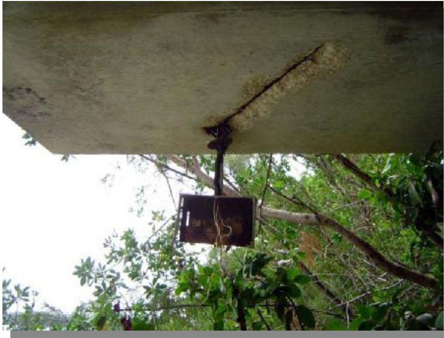
51- Conduit and Fixture Deterioration
