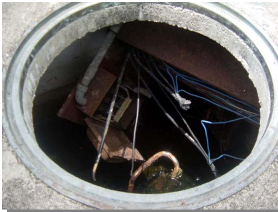
50- Lift Station Equipment Damage
