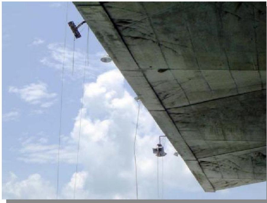
58- Lighting and Sound System Typical Condition
