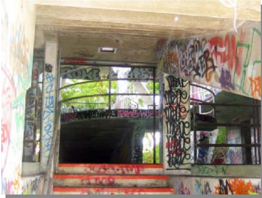
9- Ramp Area Egress with No Handicap Access
