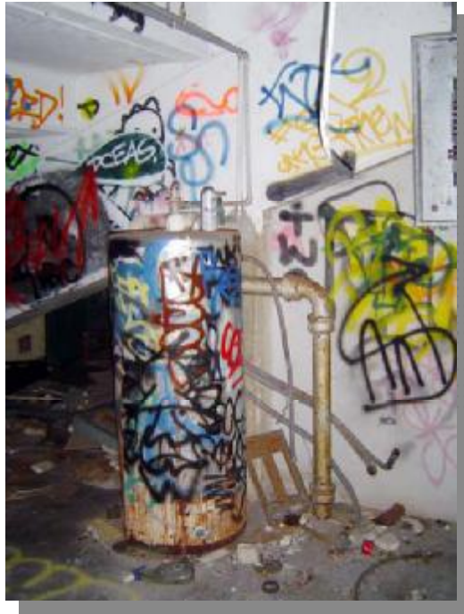
43- Water Heater and Cast Iron Piping
