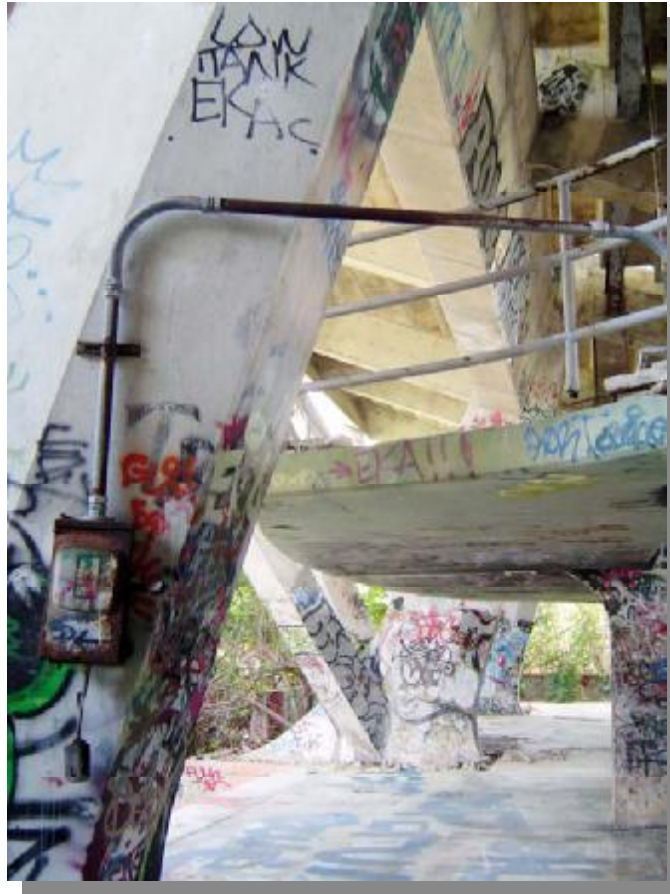
59- Electrical Disconnect Typical Deterioration
