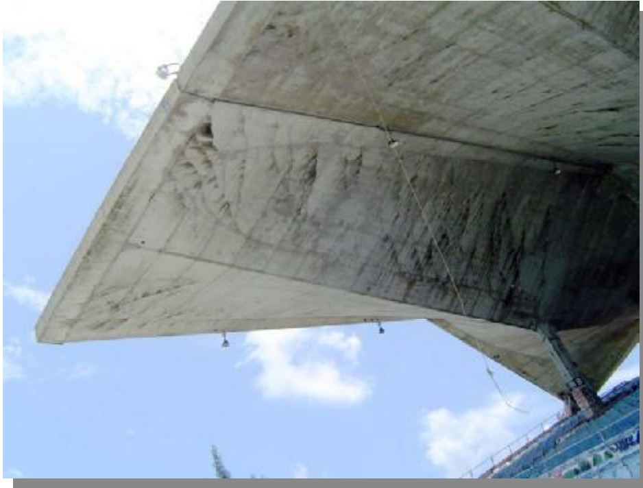
74- Over Head Concrete Structure with Water Seepage
