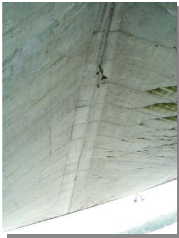
69- Over Head Canopy with Water Seepage
