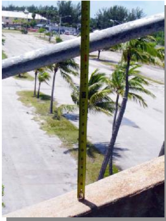
31- Railing Spacing at Grand Stand Seating Area
