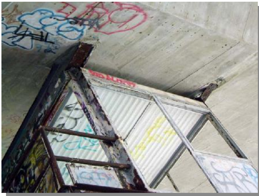
73- Control Booth Support Structure Deterioration
