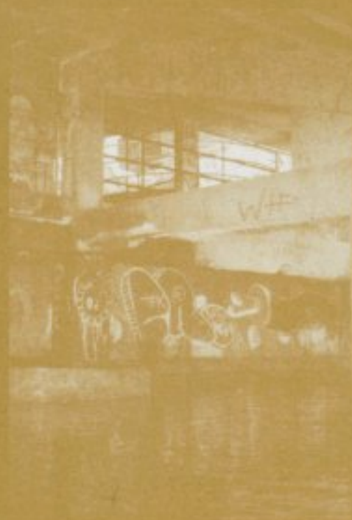
A view of the now dilapidated second-floor concourse that leads to the stadium's seating area. ©Kenneth Pietrobono
