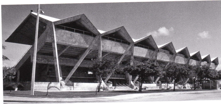
This historic photo of the Miami Marine Stadium shows the “V” shaped columns supporting the concrete cantilevered roof.
