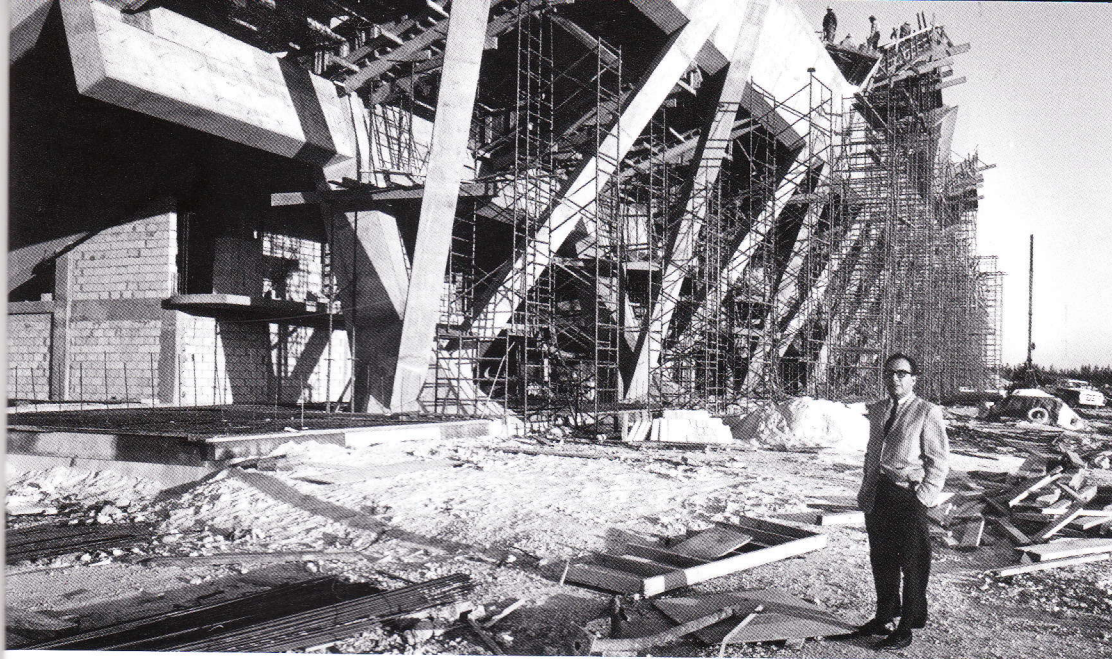
A 1963 photo shows the architect Hilario Candela standing in front of the stadium while it was under construction. In 2011, at the awards ceremony for a competition that solicited design ideas for reviving the facility, Candela notes that he never anticipated being able to look back over 50 years and “hear one of my designs, my creations, so celebrated and heartily fought for.”
